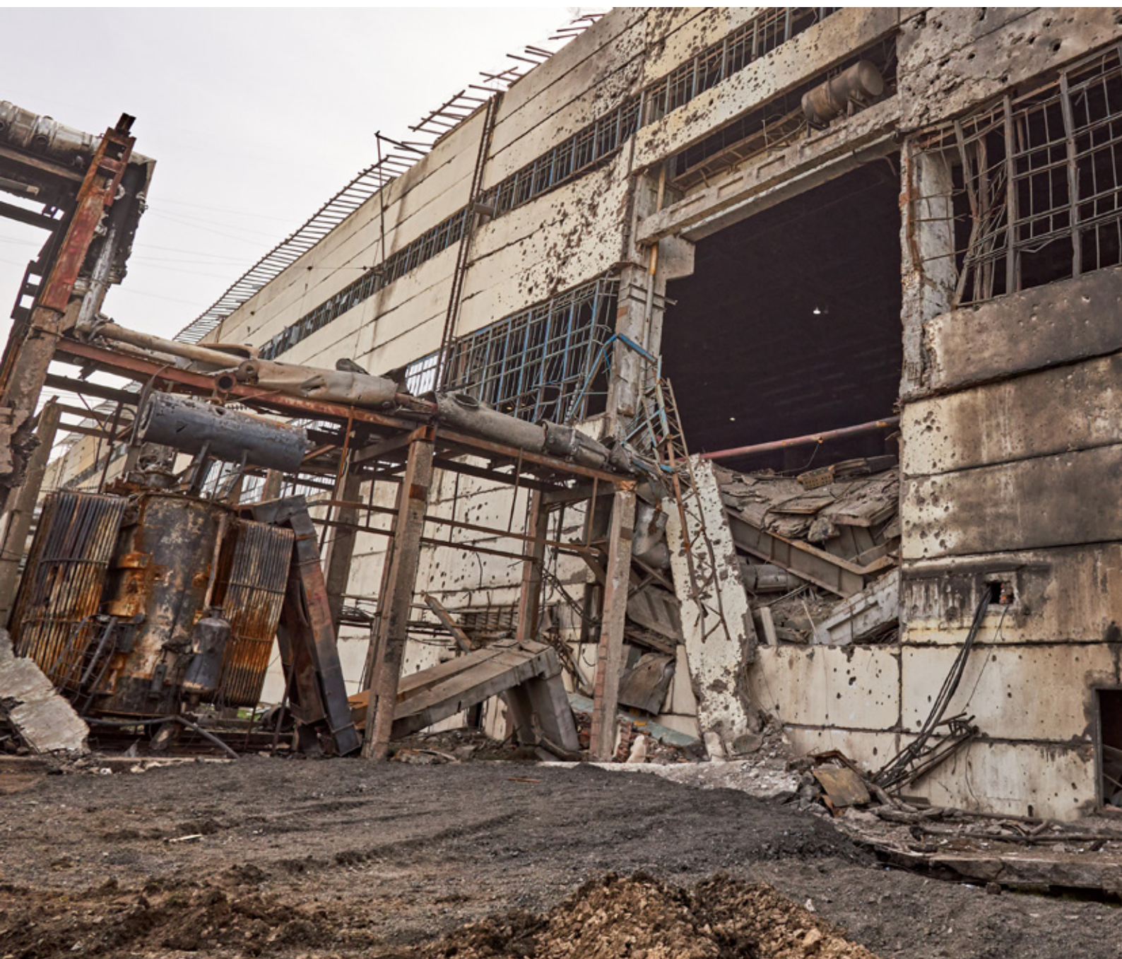
Power Plant damaged after attack. Ukraine, 2024
