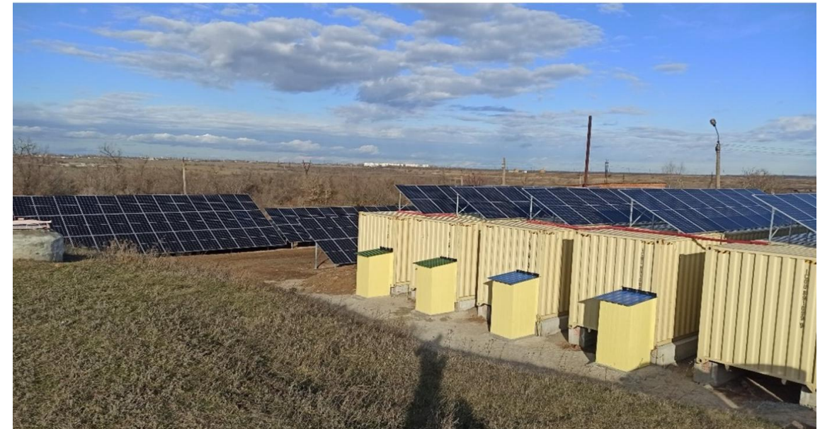
Hybrid solar power plant (PV + storage) at Mykolaiv water utility
